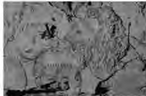
A nail, bird droppings and plaster residues
